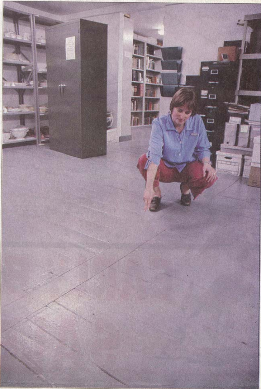
Brick Store Museum Executive Director Tracy Baetz points out a beam in the second floor that will need replacing under the museum's new capital improvement plan.
