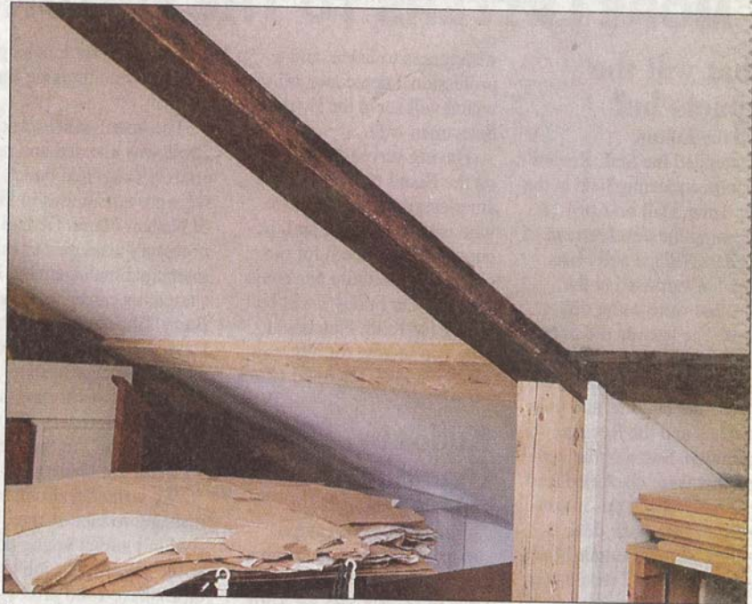
Part of the Brick Store Museum's roof has already been braced with new joists.
