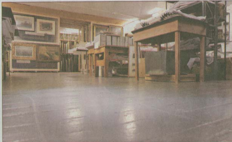
Some of the repairs needed at the Brick Store Museum are new support beams for the second floor collection storage areas, including the one photographed here. Floors are sagging and also can't bear heavy loads in some areas.
