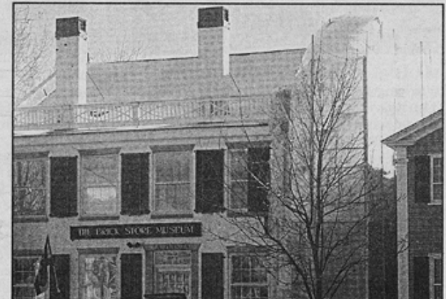
GETTING THINGS DONE - Scaffolding was recently put up outside of the Brick Store Museum in Kennebunk as part of the first phase of its capital improvement plan. (Molly Lovell photo)
