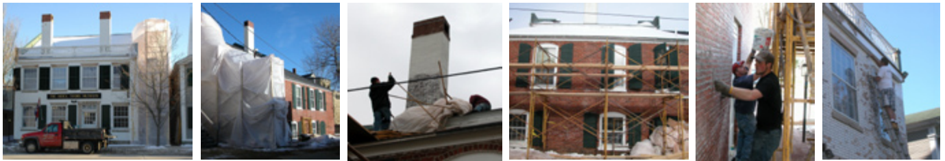
From repointing to repainting: facade and chimney restoration on the 1825 brick building.
